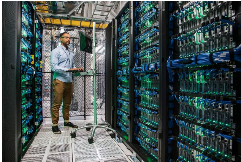
Figure. Power system reliability modeling by Infineon is offered as pivotal step towards reliable and stable power supply operation in data centers. The offering consists of an algorithm running on a digital power controller, thus integrating software and hardware. It enables real-time power supply health monitoring of the system and lifetime estimation based on dynamic system operating parameters, a power supply system model, and a reliability prediction procedure in digital power controllers by Infineon.
